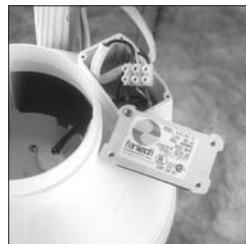
Romex wiring - Top View
